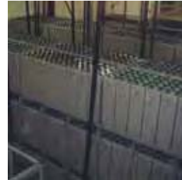
Colt Telecom in Amsterdam 24 OPzV 3000
