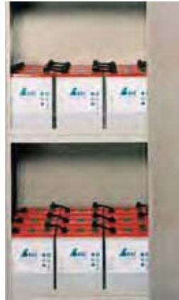
A typical compact battery system fitted into a cabinet.
