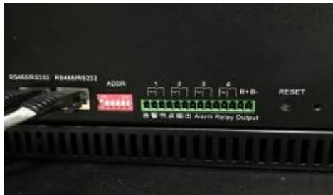
No.1 battery address:100000
