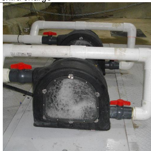
Manifold assembled on turbine
