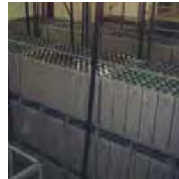
Colt Telecom in Amsterdam 24 OPzV 3000
