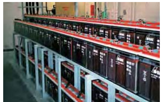
UPS application in USA 6 V 11 OGi 275
